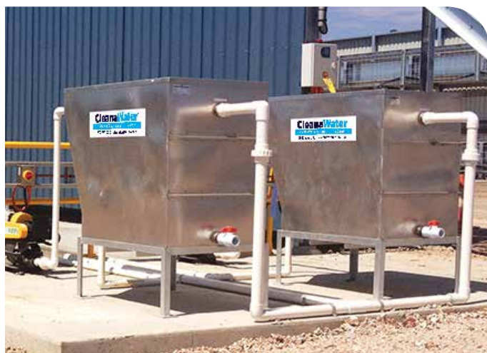
CleanaWater TS4000 SS Oil Water Separators x 2, HV Wash bay
